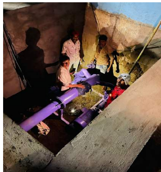
Purple pipes facilitating treated water for agriculture
