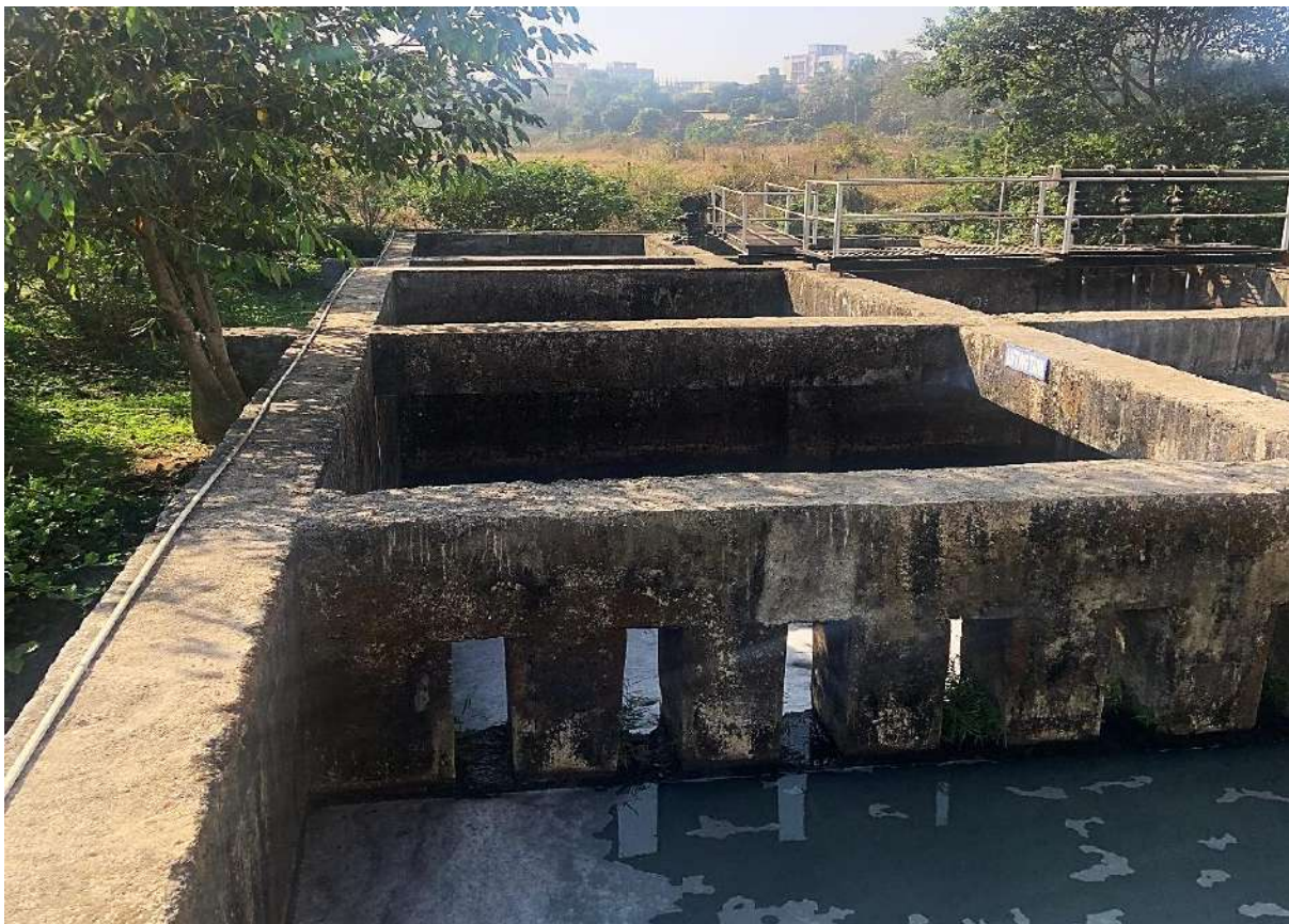
Primary treatment tank of a Sewage Treatment Plant in Dombivli, Maharashtra
